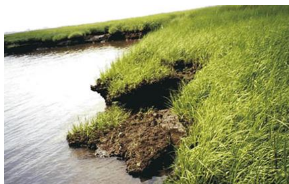
This pond bank is slumping and eroding because there is nothing holding it together except a thin layer of turf grass
